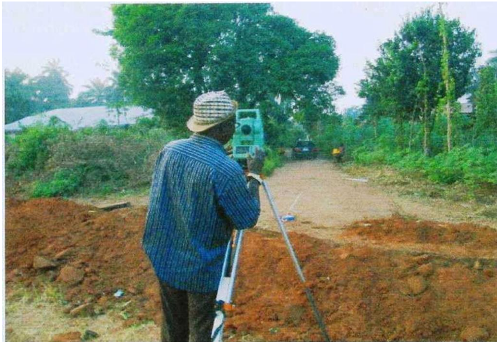
FIELD SURVEY WORK IN PROGRESS WHERE PROPOSED ROAD INTERSECTS PHASE 1 NDDC PROJECT - CH1+268
