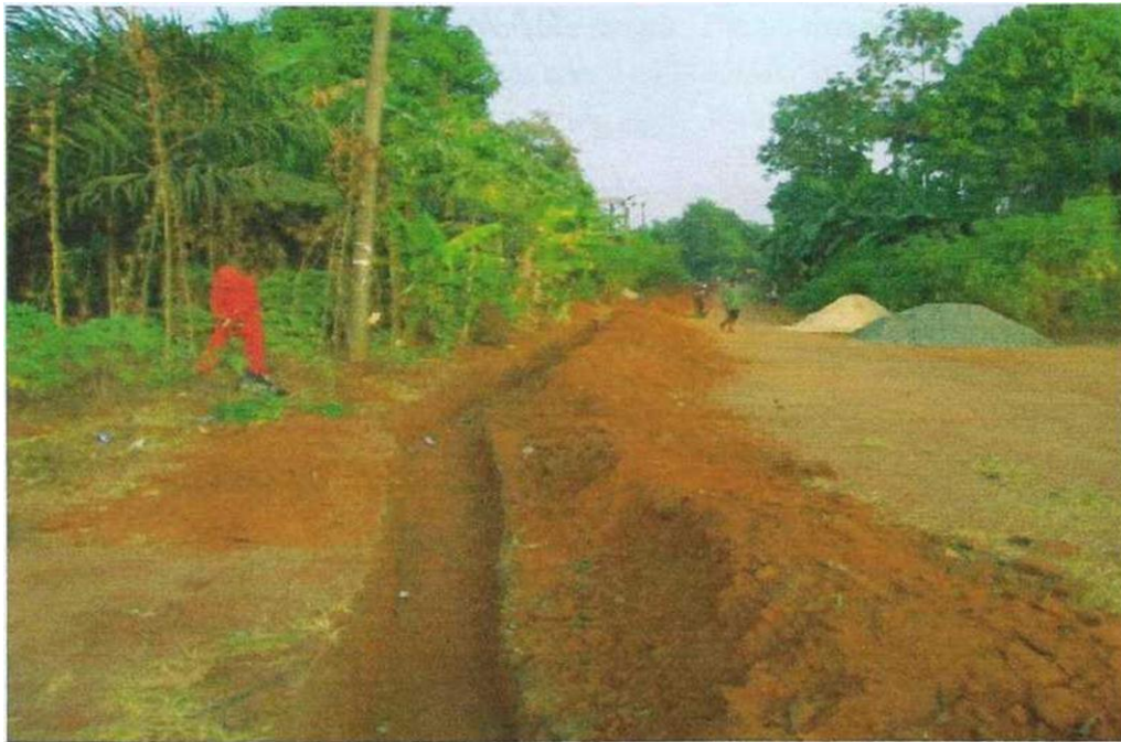
EXCAVATION FOR DRAIN ALONG NDDC PHASE 1 PROJECT AT CH 1+ 268 AT THE END OF PROPOSED PHASE 2 PROJECT
